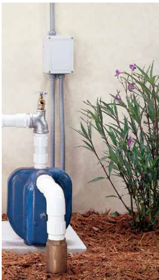
pump start relays
