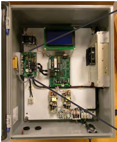
View showing all boards
